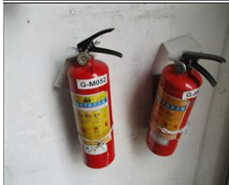
Photo of fire safety equipment 4. Fire Extinguishers.JPG
