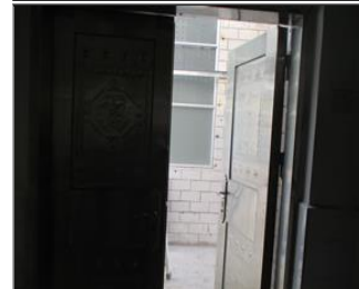
Photo of non-conformity 5. NC 7.21 Door in the kitchen is not installed with auto closed device or air curtain.JPG
