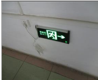
Photo of fire safety equipment 4. Evacuation Exit sign.JPG
