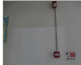
Photo of fire safety equipment 4. Fire Alarm.JPG
