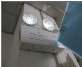
Photo of fire safety equipment 4. Testing of emergency light.JPG
