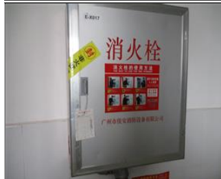
Photo of fire safety equipment 4. Fire hydrant.JPG
