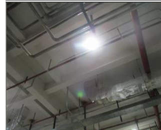
Photo of fire safety equipment 4. Spraying system.JPG
